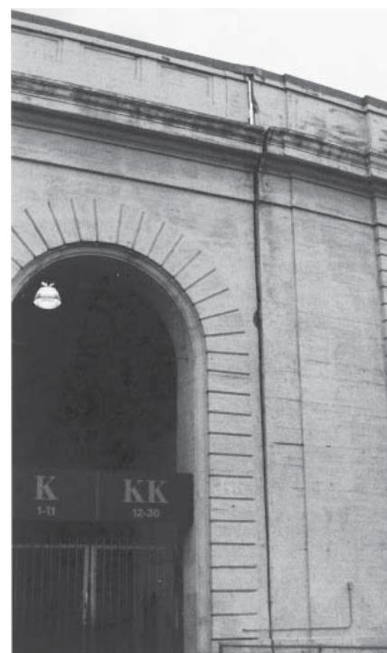
In the wall to the right of this archway in Memorial Stadium at the University of California, Berkeley, is an open crack caused by steady creep in the Hayward Fault, which runs directly beneath the stadium. From Predicting the Unpredictable .
